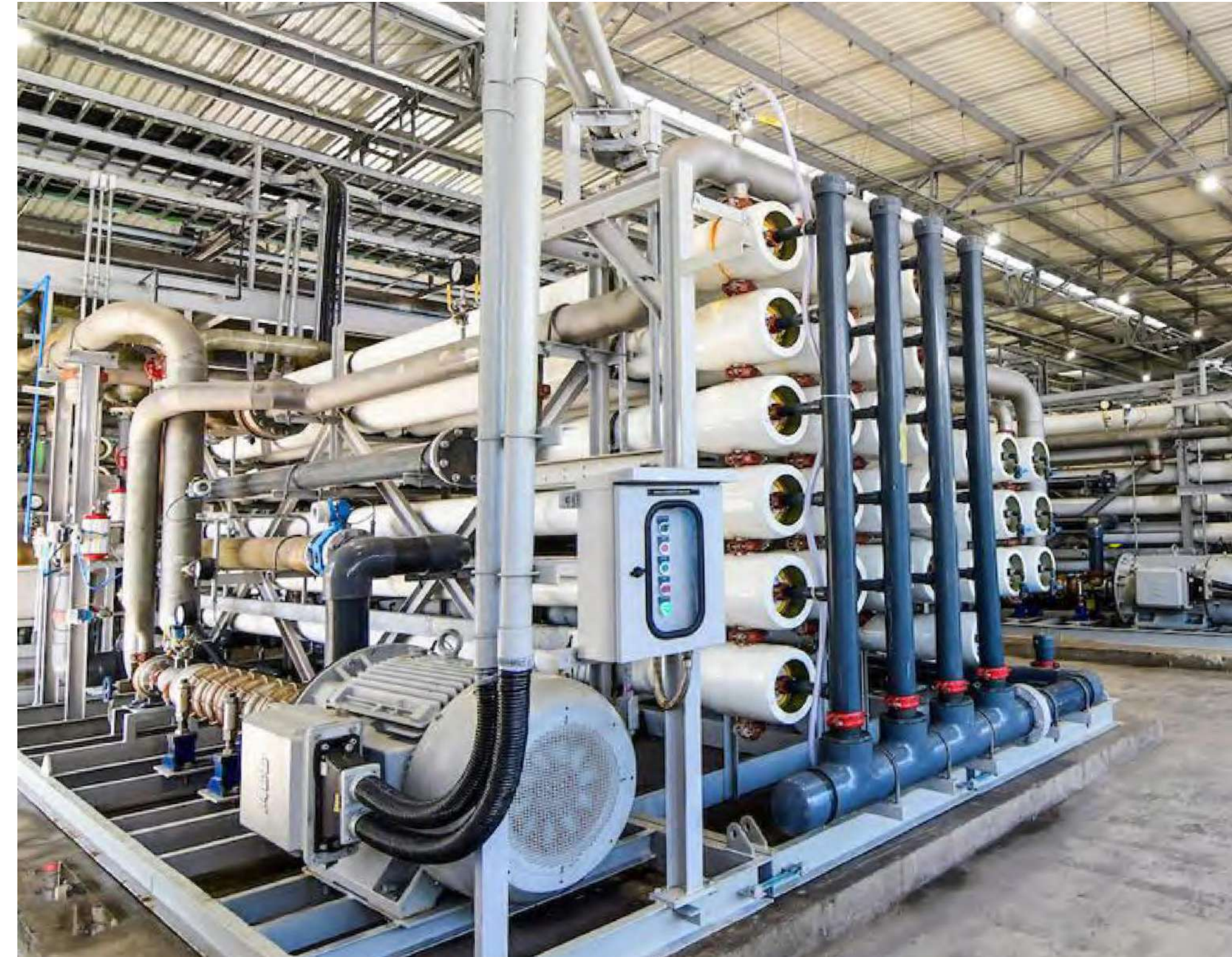
Desalination plant located at the Tubarão unit, in the State of Espírito Santo, is part of the Water Master Plan
